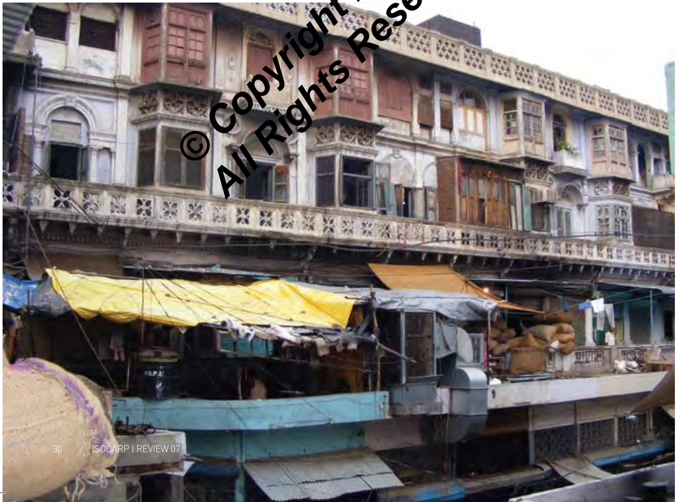
Figure 7: Inner-city housing above the spice market in Shahjahanabad, Delhi Photograph © Marina Faetanini, courtesy UNESCO New Delhi
