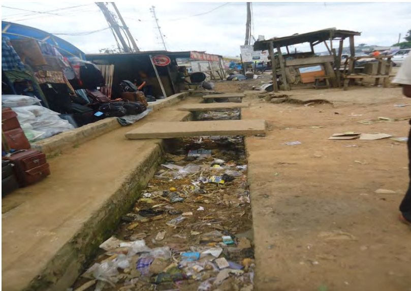
Plate 4.1: Silted drainage at Sabon-Gari during dry Season
