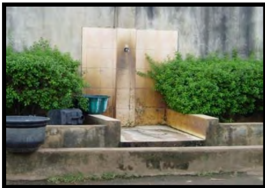
Photo 5: Borehole water point outside a house
