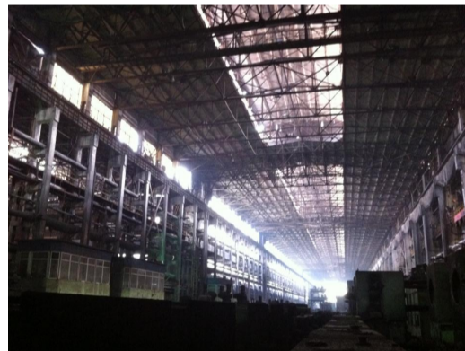
Figure 12: Use of large roof area of industrial building for solar panels
