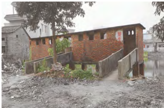
Figure 1 Restroom without sewage system
