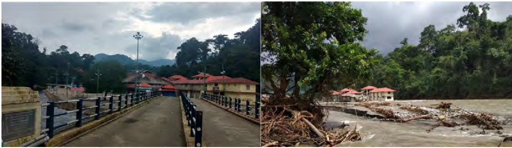
Figure 9. Before and after flood - Bridge
