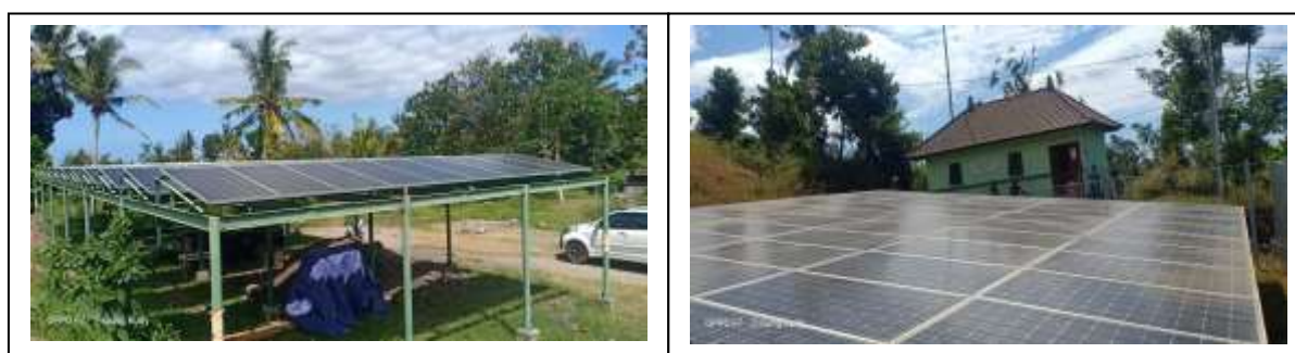
Figure 6. Solar Power Plant 23 kWp in Klungkung for irrigation and 10 kWp in Karangasem for electricity for 18 households & 3 public facilities. Source: Field Survey 2020.
