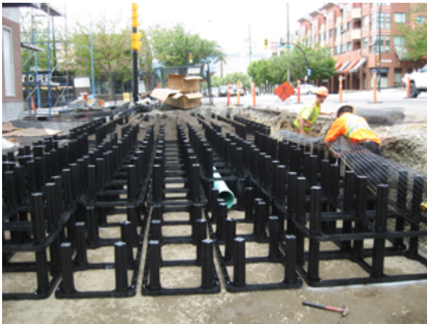
FIGURE 17: Soil cells can be used to provide additional soil volume for trees on sites that need to support heavy weights such as vehicles. This site in the City of North Vancouver is using silva cells to provide more soil for tree roots to grow into. Stormwater from the street is being redirected into the soil via an adjacent catch basin. Excess water is captured by a drain line at the bottom of the cells connected to a downstream catch basin.
