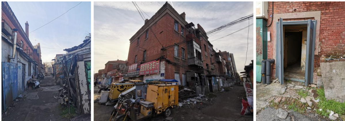
Figure 2 The pavement and roadway are in disrepair and piled up with waste. Source: author.
