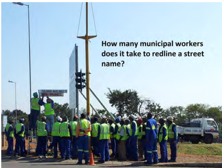
Figure 2: Changing street names in Tshwane, workers being trained on how to put up the new street names and 'red-line' over the old names. Photo by M v d Vyver (City of Tshwane)
